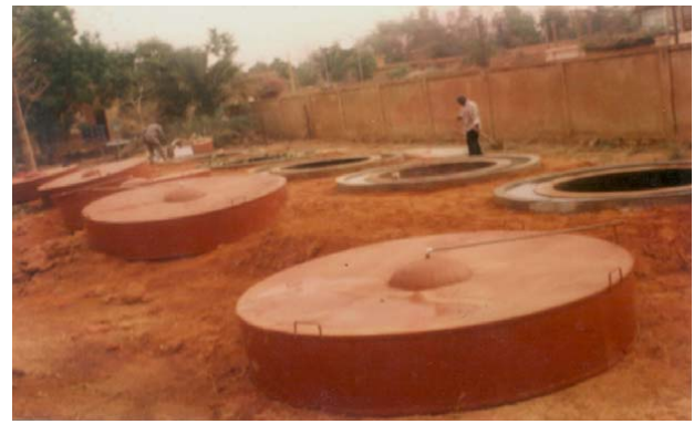
Figure 1. View of production digesters.
